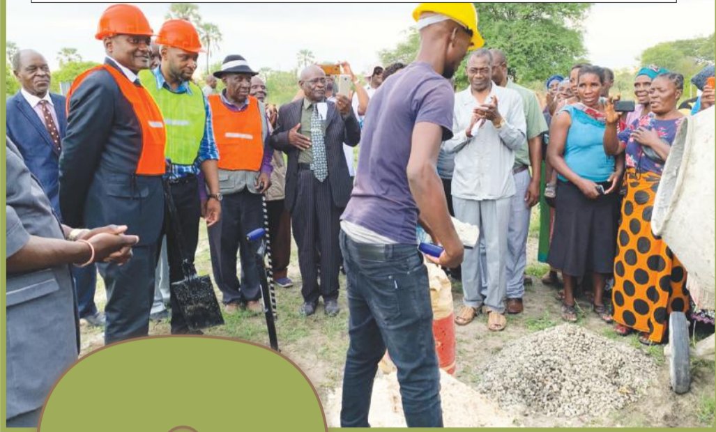
Ground breaking ceremony of the Lusese Climate Resilient Infrastructure (Flood Relief Centre) under the CBNRM-EDA Project. Hon. Pohamba Shifeta, Minister of Environment and Tourism and Mr. Benedict Libanda as seen with the beneficiaries of the Lusese Village, Zambezi Region.
